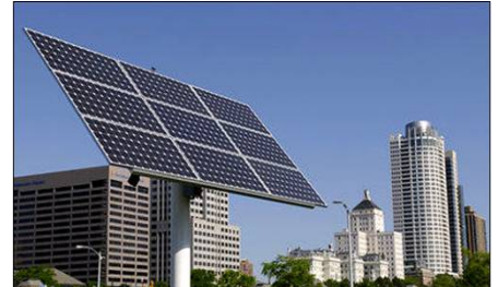
Solar Electric Ground-Mounted Solar Array at Discovery World
