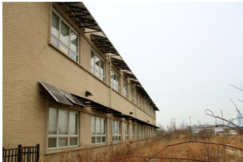
Figure 7: At the Chicago Center for Green Technology, solar panels serve a dual purpose, as they are used to generate electricity and are used as awnings above windows. This is an example of a non roof-mounted system. (Source: http://news.medill.northwestern.edu )
