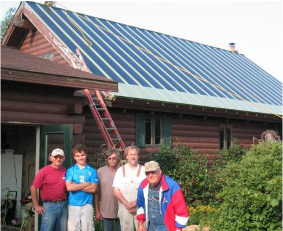
Photo 2. Standing seam metal roofing with 3.5 kW of integrated solar electric modules on an older home in Edgar, Wisconsin (photo credit: Lake Michigan Wind and Sun).
