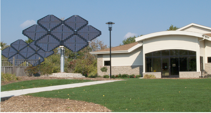
Photo 5. Two attractive ground mounted solar electric system, with a capacity of 2.1 kW each, located at Northeast Wisconsin Technical College. This system won and Mayor of Green Bay's Beautification award (photo credit: Lake Michigan Wind and Sun).
