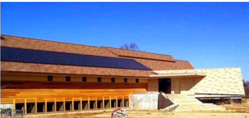
Photo 4. 8.5 kW of SunSlates® on the roof of the University of Wisconsin's architecturally significant Arboretum Visitor Center addition. Slates could have been used to roof the area around the solar electric system, but to save on cost asphalt shingles were used (photo credit: UW Arboretum).
