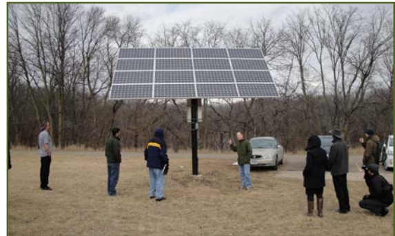
Ground Mount System, CERTs
